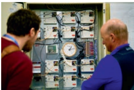
A view of the central clockwork mechanism in the basement of the Palais des Nations.
