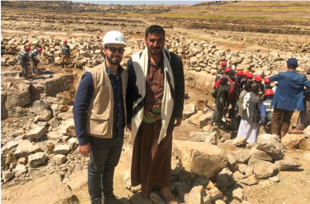
Mohamad Marji (WFP, left) with cooperating partner staff supervising the progress of a rural road rehabilitation project in Sana'a Governorate.
